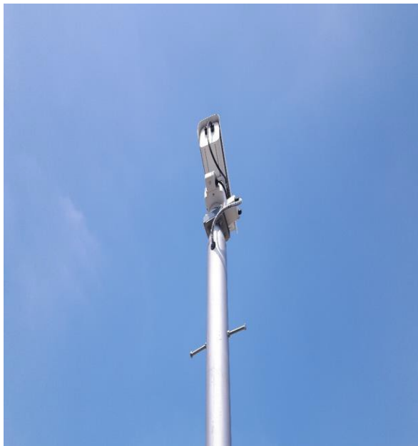
Fire response camera pole
