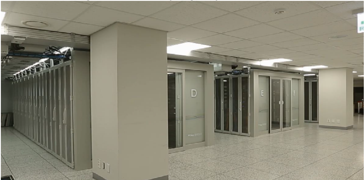
Figure 19. IFEZ Smart City Integrate System SDDC Center
