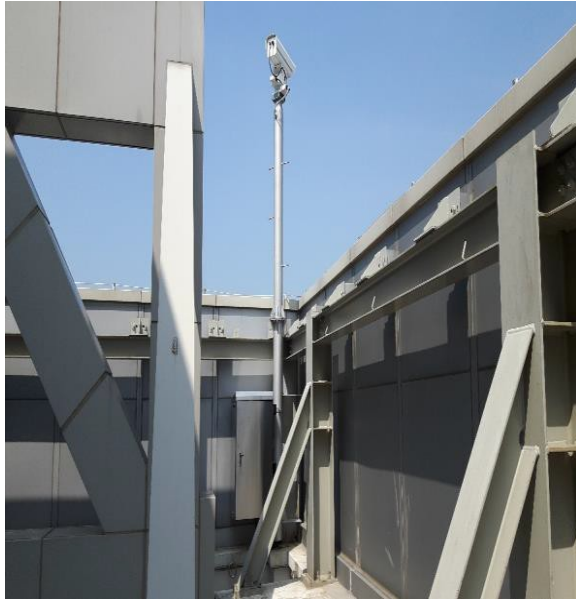
Fire response cameras (installed at G-Tower)
